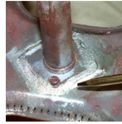
Pyro-Putty® 653 seals corroded burner manifold.
